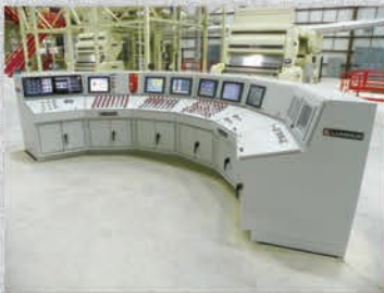
Controls and Control Systems
